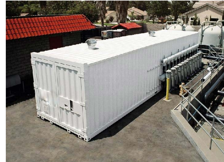
1,000-GPM Perchlorate Removal System - California
